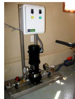
Backwash recycle pump skid
