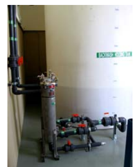
Backwash Filter, Tank
