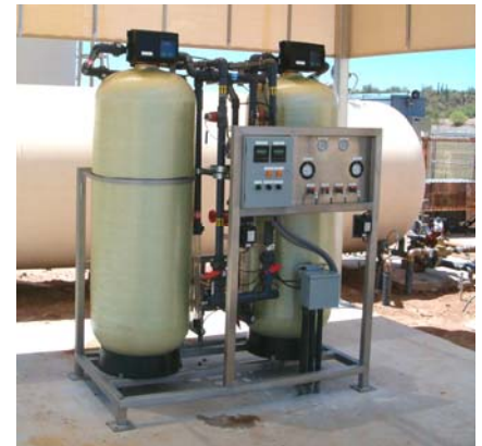
APU-30 System – New River, AZ Arsenic Treatment Project
