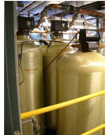
Clarkston, Michigan Arsenic Treatment System installed May, 2003
