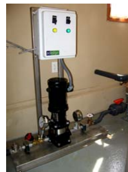
Backwash recycle pump skid
