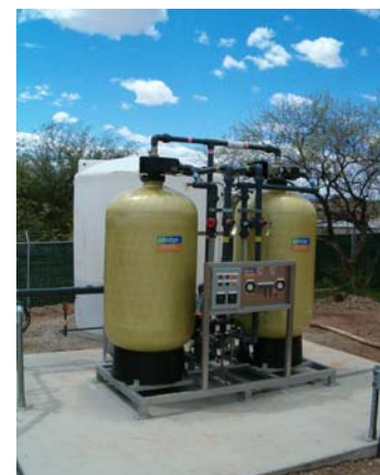
APU-25LL System – Carlin, Nevada Arsenic Treatment System
