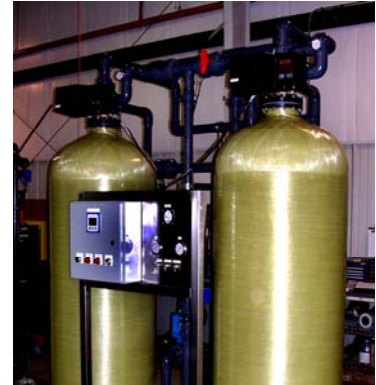
APU-25LL System – Carlin, Nevada Arsenic Treatment System
