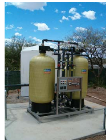
APU-100 System – Rimrock, Arizona Arsenic Treatment Demonstration
